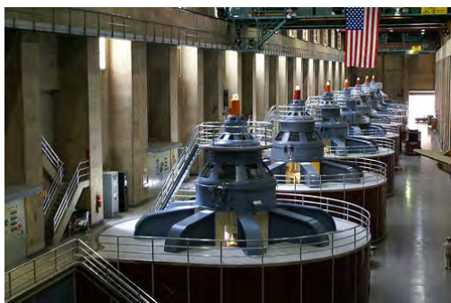
The generators inside the hydroelectric power plant.
